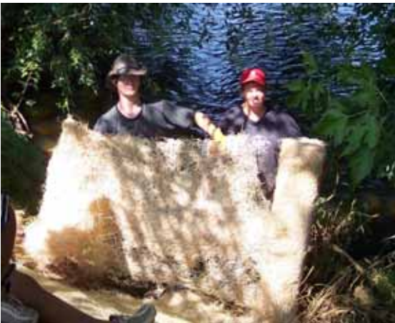
Fiber matting was cut and laid around the rock to help hold grass seed.
